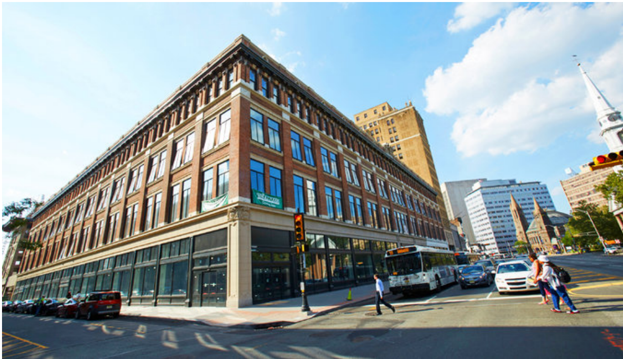
The former Hahne’s department store is undergoing a restoration that will transform the structure into 160 apartments, a cultural center for Rutgers University and a Whole Foods Market. Alex di Suvero for The New York Times
